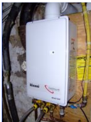
Rinnai tankless water heater warning code for lime deposits appears after 5 months
